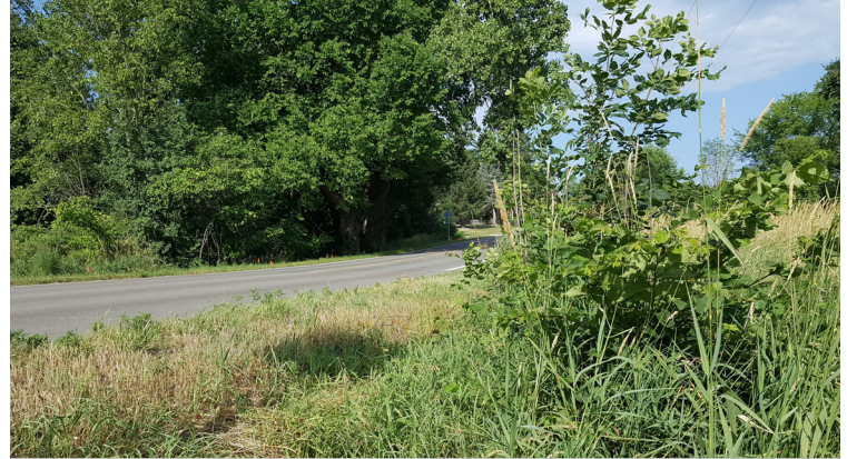
An example of overgrown roadside vegetation that will be sprayed with herbicide
